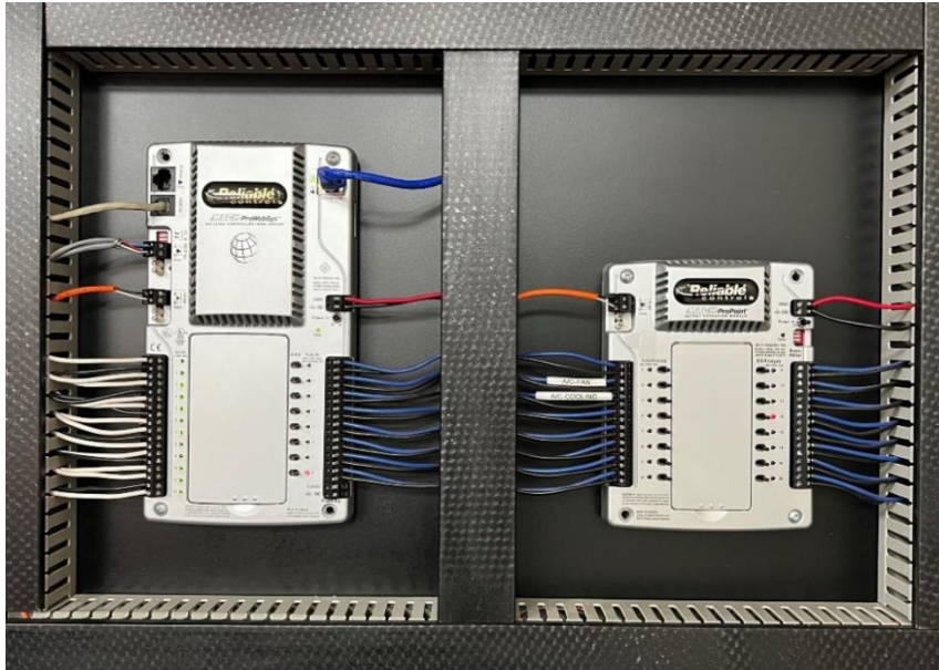
Figure 2: Direct Digital Control (DDC) System Panel
